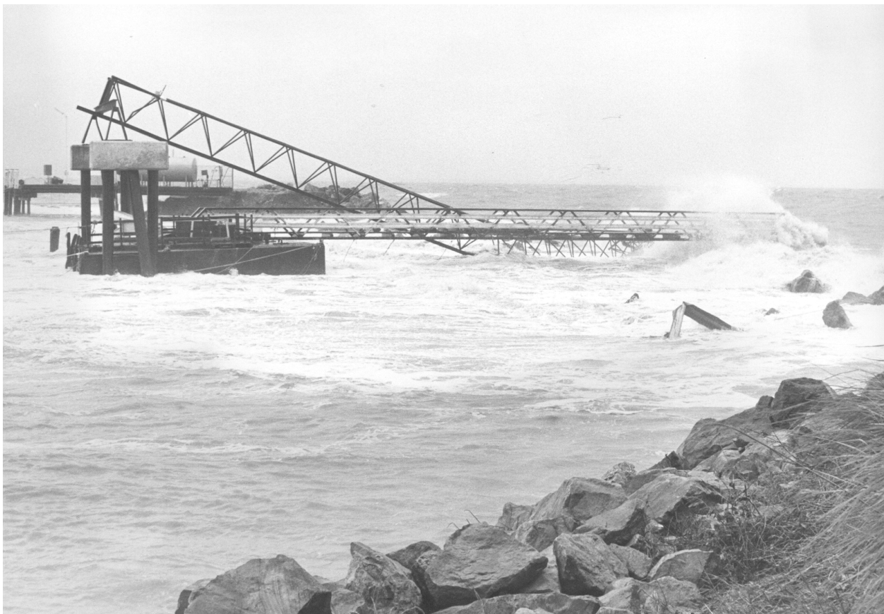
Figure 2 Large seas combined with high tides caused considerable damage to breakwaters, retaining walls and other structures especially at Rosslyn Bay Harbour (above) where the Breakwater was destroyed along with yachts and trawlers.
